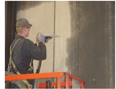
fire damage - soot on concrete
