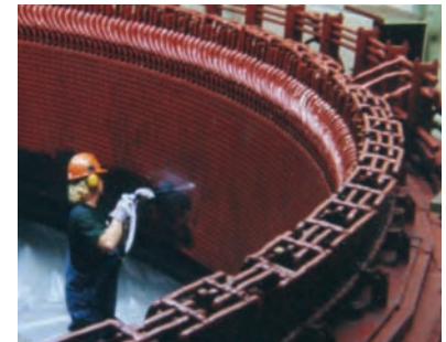
electrical - generator cleaning
